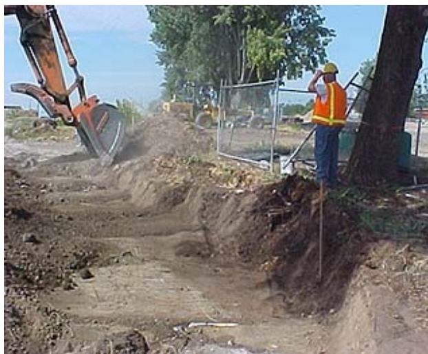
This excavation cut a tree's roots, a costly mistake that could have been avoided!
