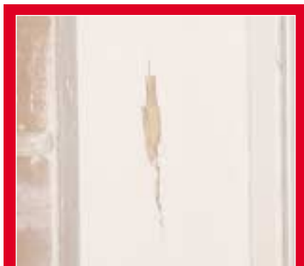
Figure 1: Drywood termite damage
